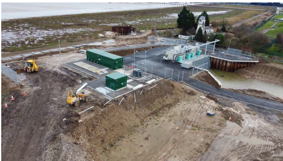
Figure 1-3: Aerial Photograph of the AMEP Surface Water Pumping Station
